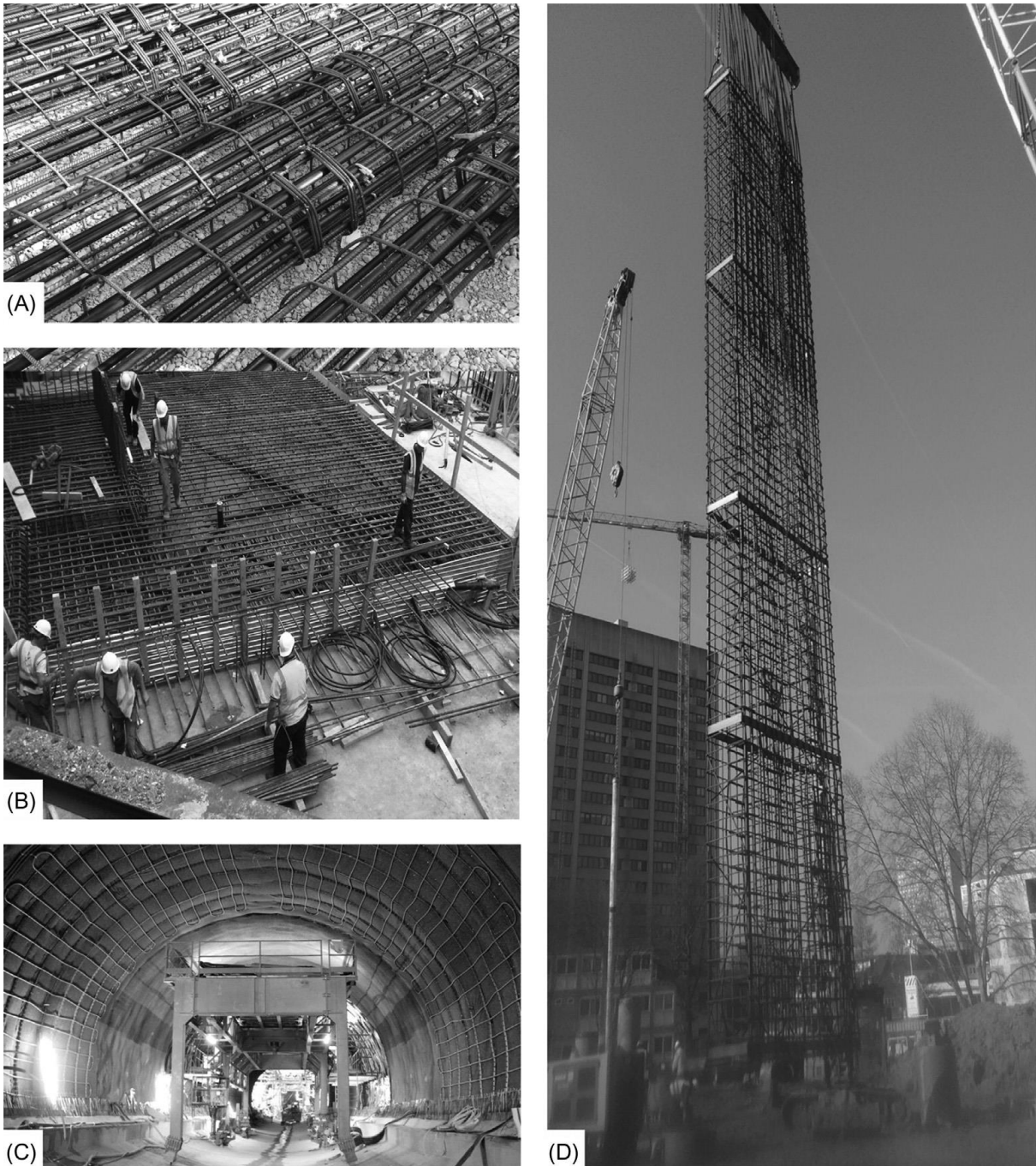
Figure 2.10 - Heat exchanger pipes installed in a) energy piles, b) energy slabs, c) energy tunnels and d) energy walls, (Laloui & Rotta Loria, 2020).
